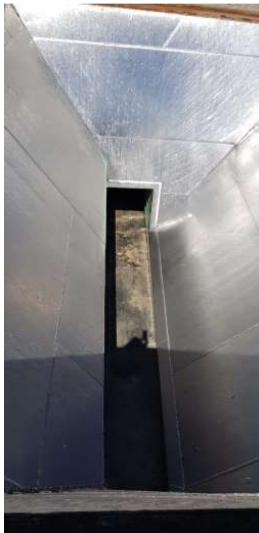
Detail of Hopper state before the manufacture of the new wall and the tunnel with MTS
