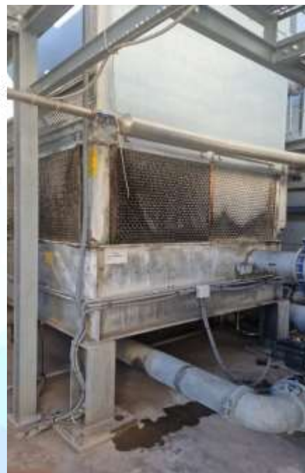
Outside of Cooling Tower.
