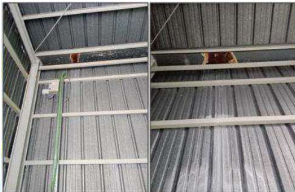
Detail spouts corrosion and loss of section that caused leaks.
