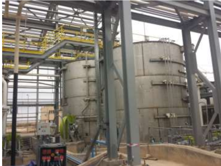
Stainless steel storage tanks of amide before action
